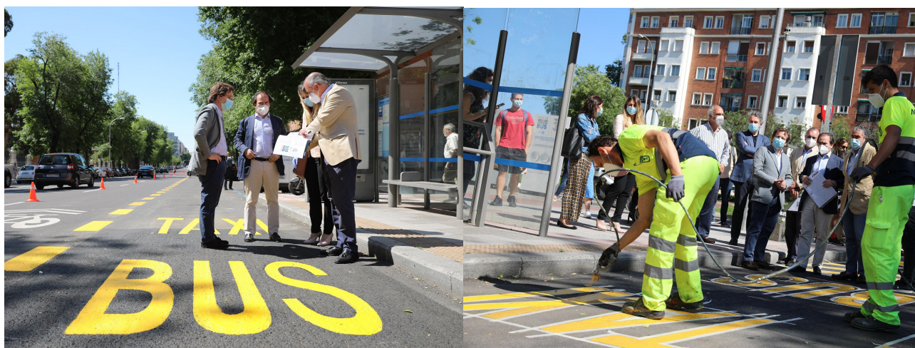
Figure 13. New pop-up bus lanes (marked in yellow) implemented in May 2020 which have been turned into permanent ones by November 2020
